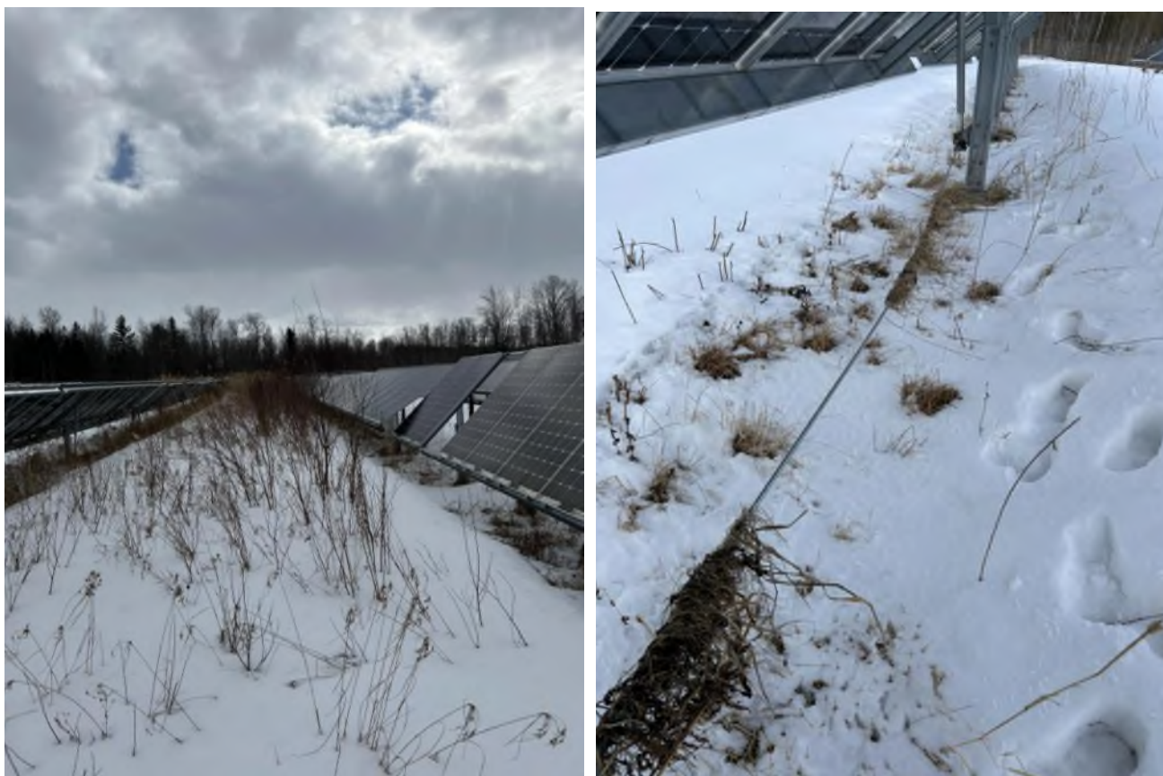
Figure 6-13 Vegetation overgrowth across site
