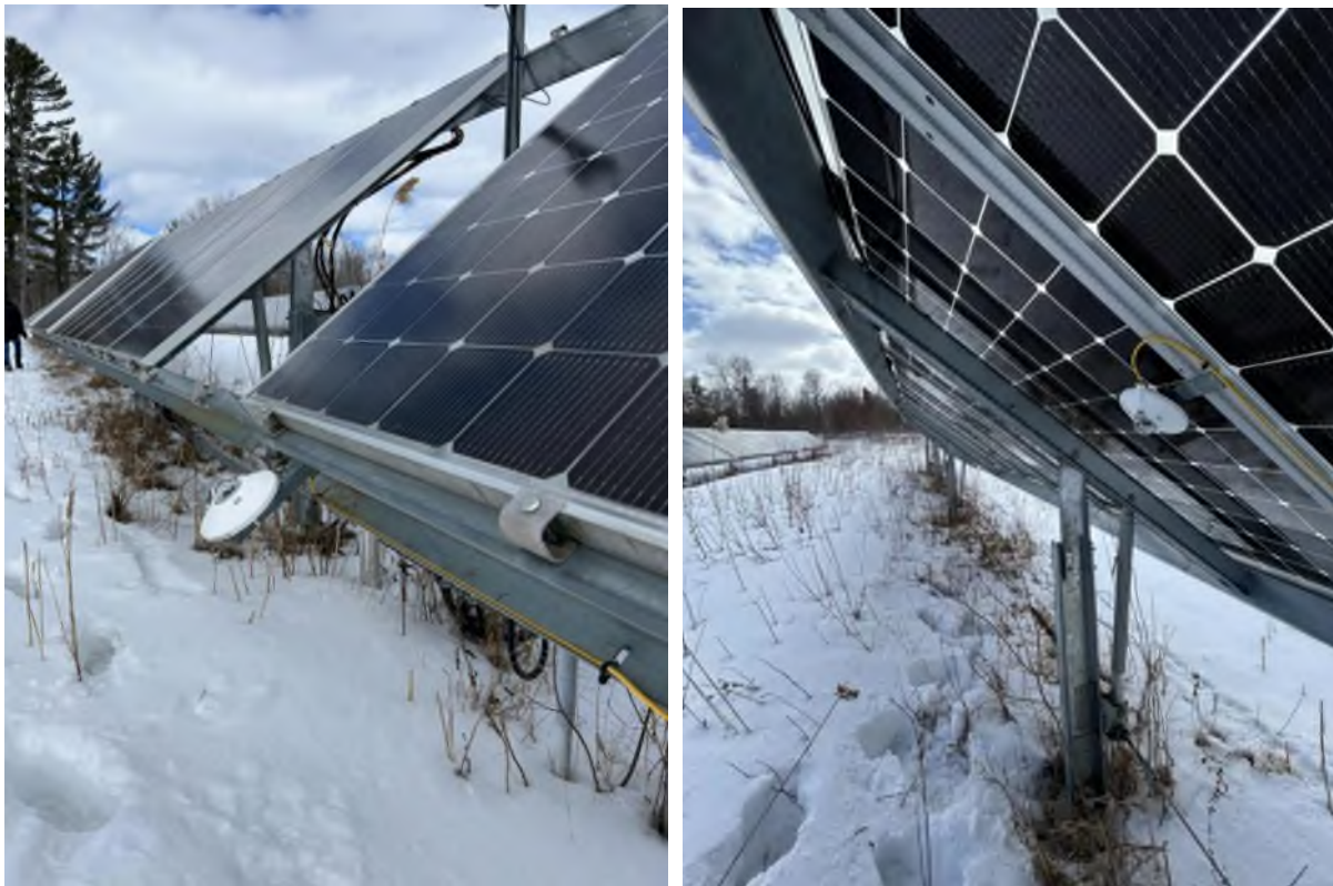
Figure 6-14 Pyranometer installed on row #1
