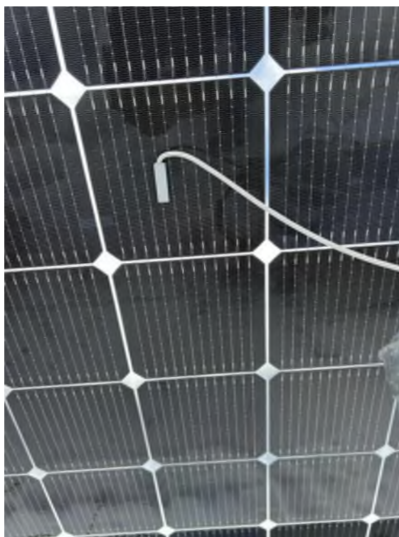
Figure 6-15 Module temperature sensor installed on row #1
