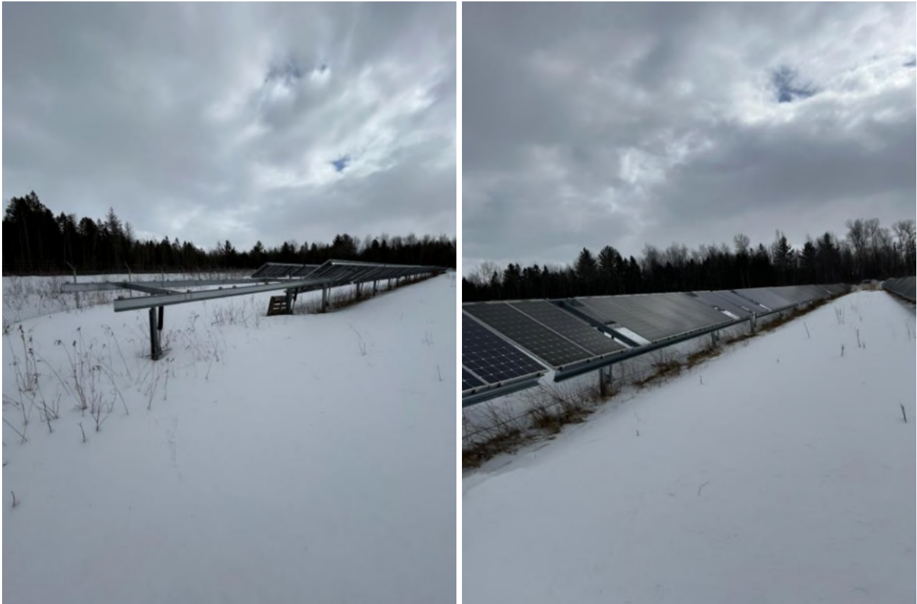
Figure 6-7 Missing modules observed across the site
