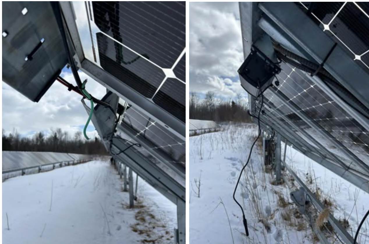
Figure 6-10 Damaged ground cable, tracker motor cable not connected
